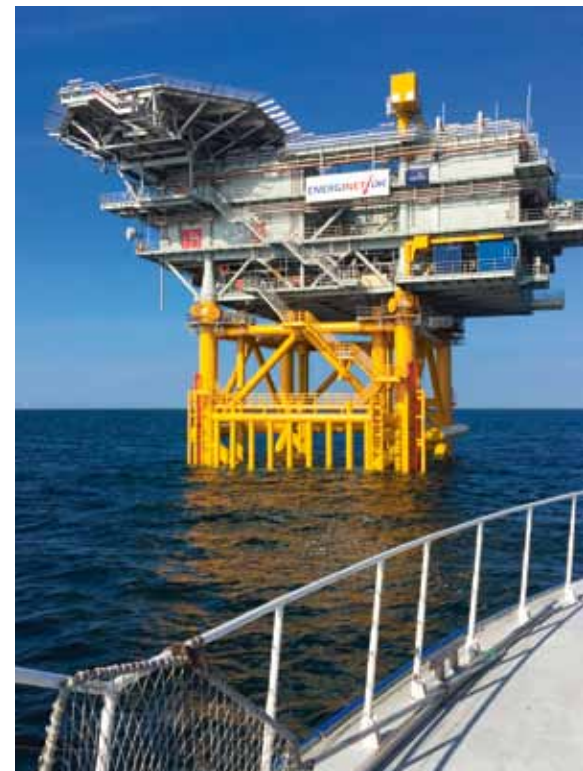
Offshore high voltage substation at Horns Rev C offshore wind farm.
