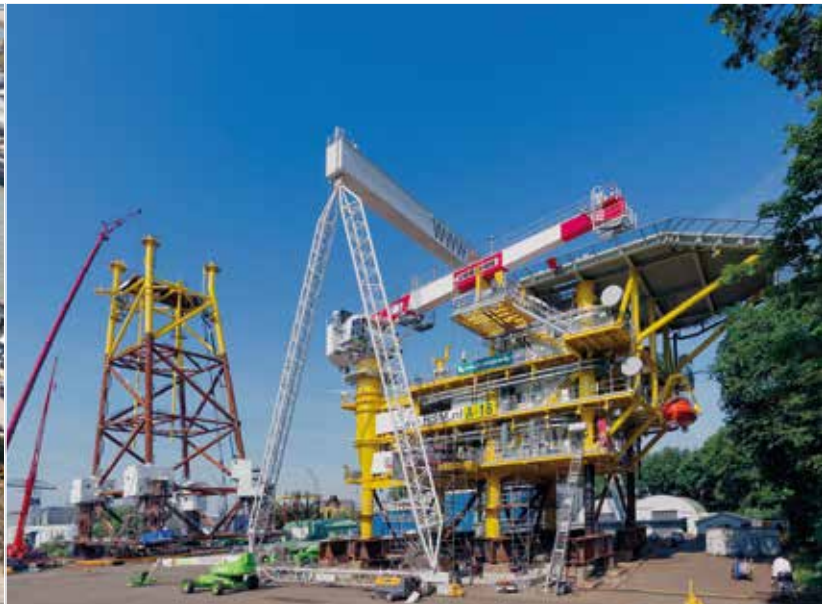
EPCI gas platform
